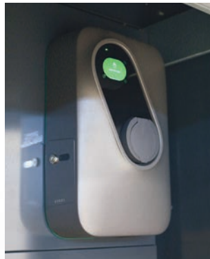
Integrated EV charging points
